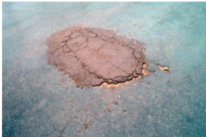
(c) Remendo mal executado (R)
